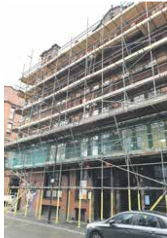
Maintenance package for Daresbury Science Technology Park and ongoing works for the National Trust on Speke Hall and Chambre House in Liverpool.
